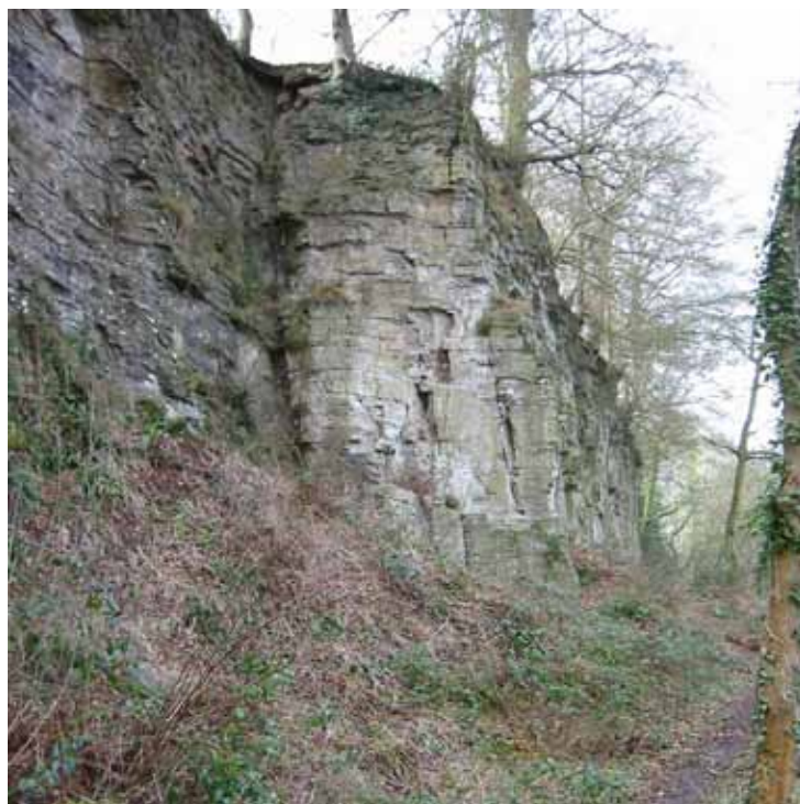
Stress relief fractures visible at Whitcliffe Quarry © Michael Rosenbaum
