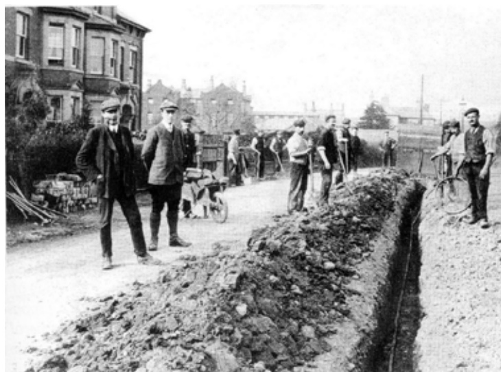
Trench being dug on Gravel Hill (1905) From 'Victorian Ludlow' published by Ludlow Historical Research Group
