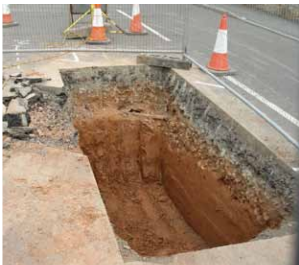
Roadworks on Whitefriars reveals the sand deposit immediately beneath the surface © Michael Rosenbaum
